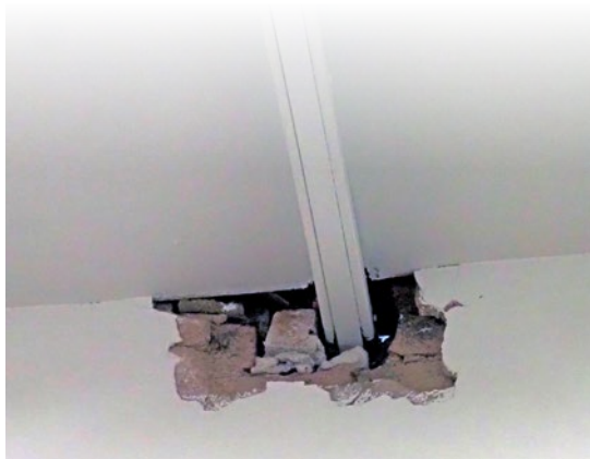
The room has gaps round pipes or by the ceiling thus compromising its fire integrity.
